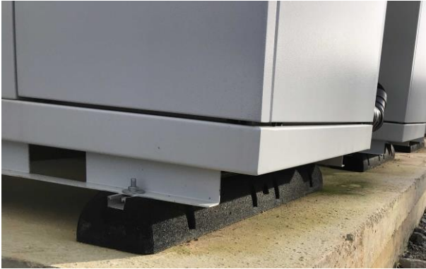
Figure 55: Unit mounted on concrete slab with anti-vibration pads
