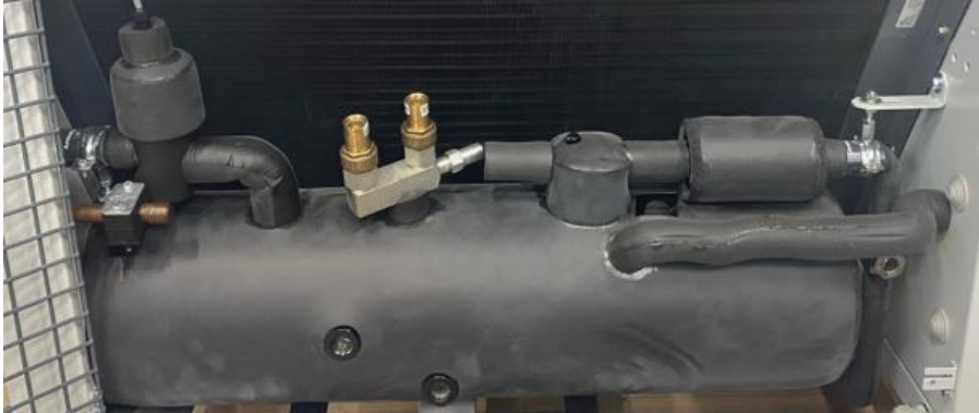
Figure 43: Liquid receiver with safety group
